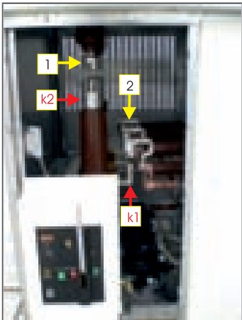
Circuit breaker position: DISCONNECTED
