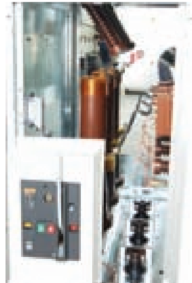
Cable Compartment of Cubicle with Circuit Breaker
